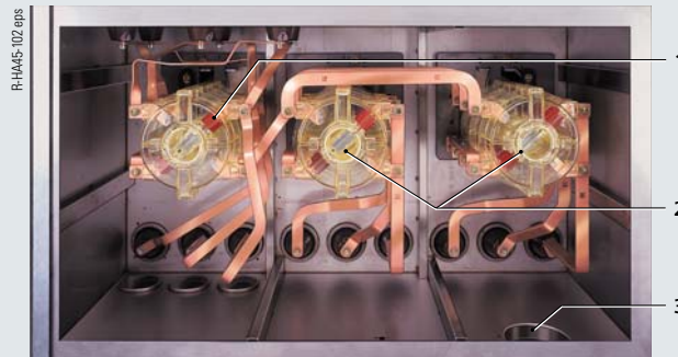
Switchgear vessel of a ring-main/transformer block, scheme 10 (rear view)
