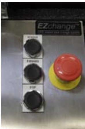
Control panel for soft start
