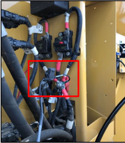
Figure 14: Cable C30 Power Connections
