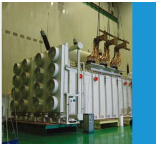
沈变——华润湖北 SFP-1140MVA/500KV Shenyang transformer-Huarun of Hubei province SFP-1140MVA/500KV SFP-1140MVA/500KV
