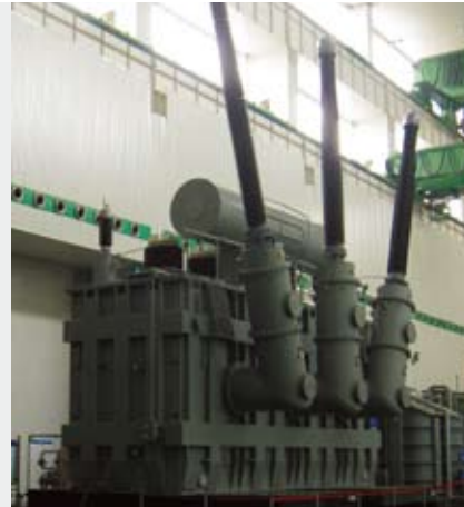
衡变——湖南宝庆电厂 FSP-780MVA/500KV Hengyang transformer-Baoqing power plant of Hunan province FSP-780MVA/500KV
