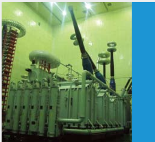
衡变——溪洛渡水电站 SSP-860MVA/500K Hengyang transformer-Xiluodu hydropower station SSP-860MVA/500K
