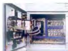
D 继电器仪表室 Relay instrument chamber
