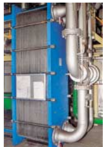
Process water heating in the food industry
