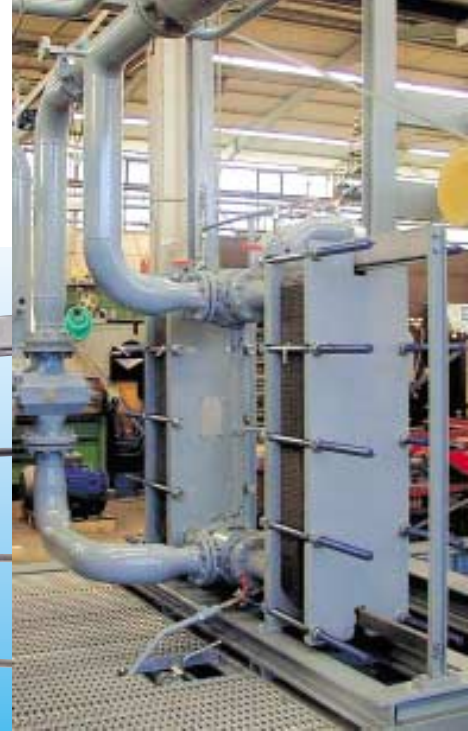
Double oil cooler in a power plant
