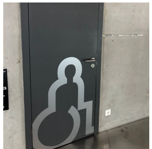
The door to the accessible toilets on floor three of petal, the door is particularly heavy and does not have an automatic open button
