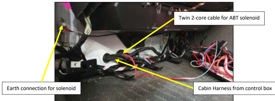
Figure 19: Connection for interface cables back of fuse board.
