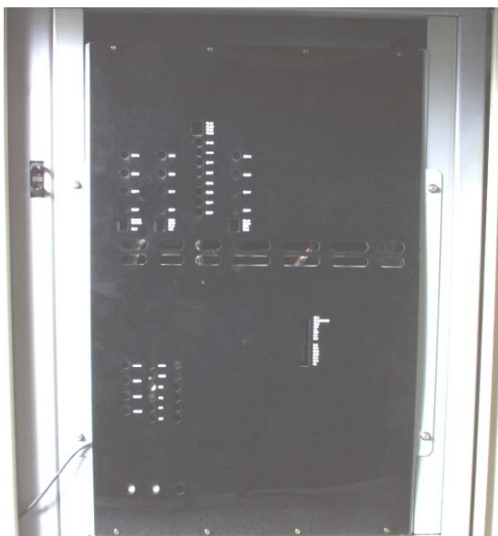
Fig. 4.6 Control panel R2
